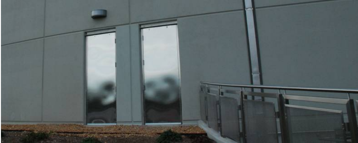
Figure 3-4 Emergency Exit Doors
